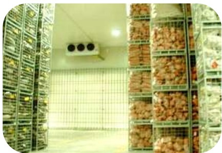
Absence of energy efficient cold storage techniques
